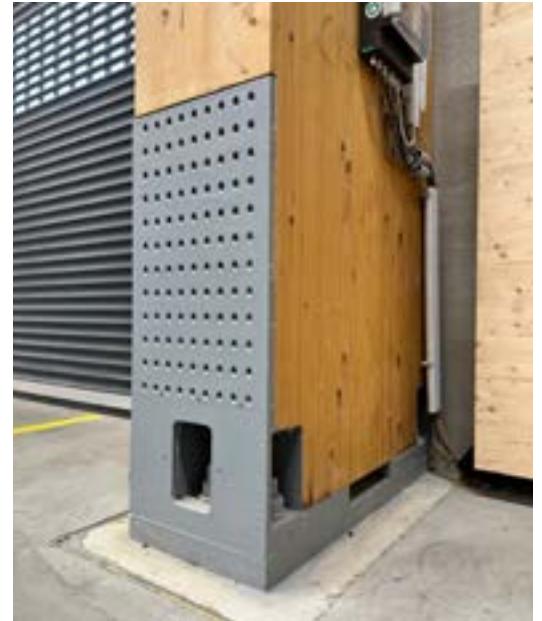
Detail pin-ended column primed and R30 fire protection coated. Top coat RAL 7001 in the visible area.
